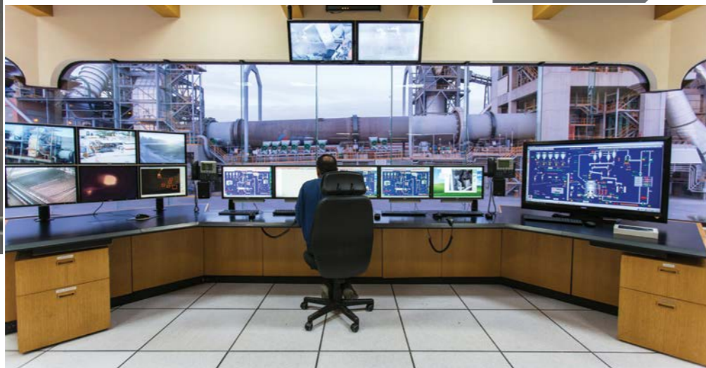
↓ Sala de control Planta Samalayuca. Samalayuca's Plant control room.
